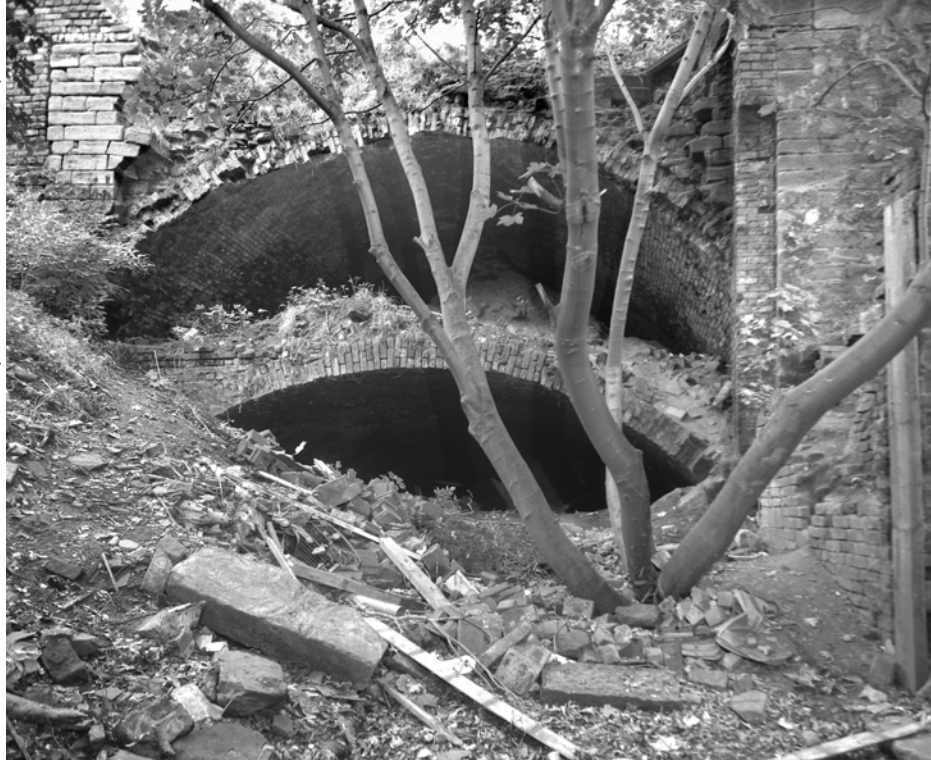
Williamson's double tunnel in the stable yard at Smithdown Lane in 1998 before restoration Photo Nick Catford
